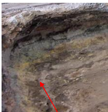
Localized cathode corrosion evident at pot corner from extended bath toe
